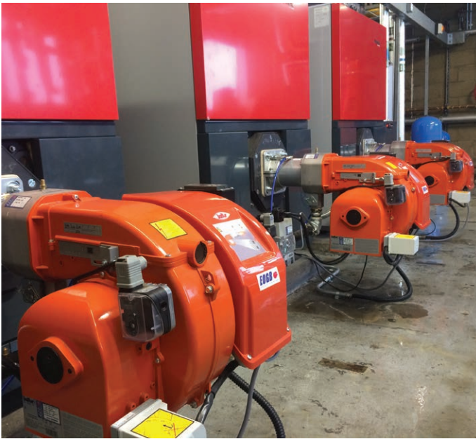
EOGB installed three Baltur TBG 45PN gas burners at Ashford International Station
