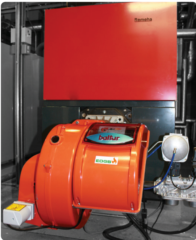
The improved heating installation at the City of Bristol College is highly-efficient and makes use of the latest technology
