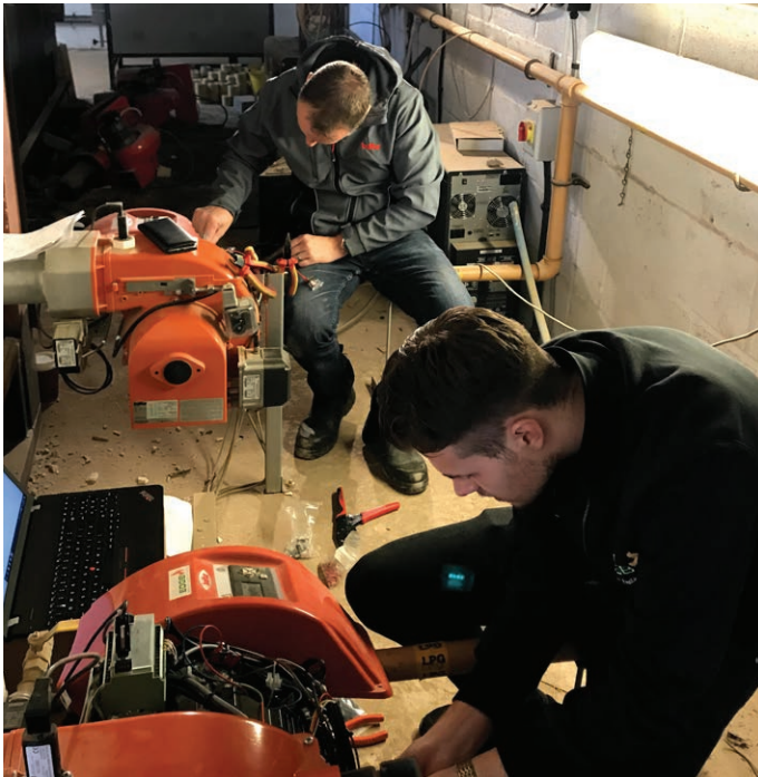
The new burners installed at H.G Matthews incorporate custom PLC controls which have significantly improved production yield
